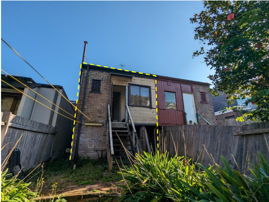
Figure 7: Rear of subject dwelling (outlined yellow) viewed from rear yard facing northwest
